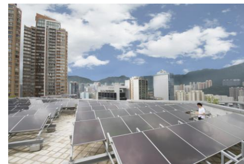
Building-integrated PV panels on Trade and Industry Tower in Kai Tak
