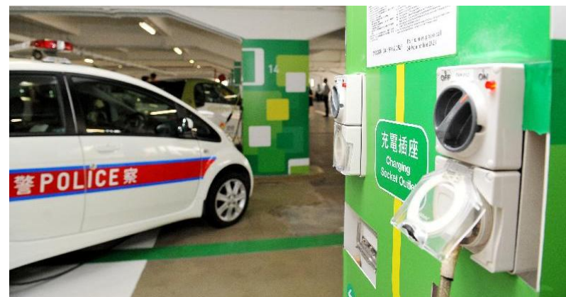
Figure 6.8 EV charging point at government car park Source: Information Services Department
