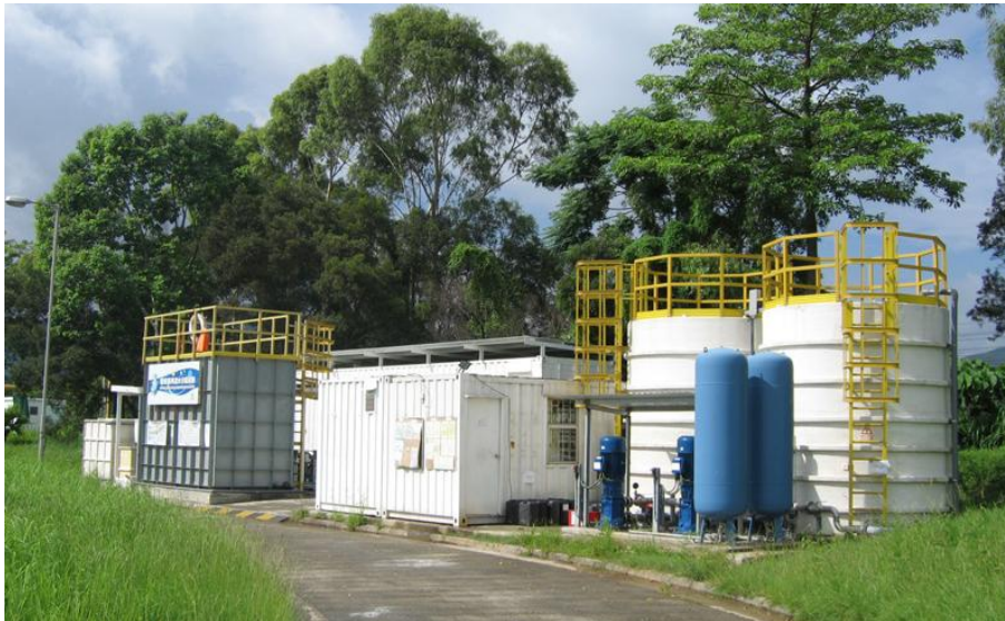
Figure 3.8 Reclaimed water treatment plant in Shek Wu Hui Sewage Treatment Works
